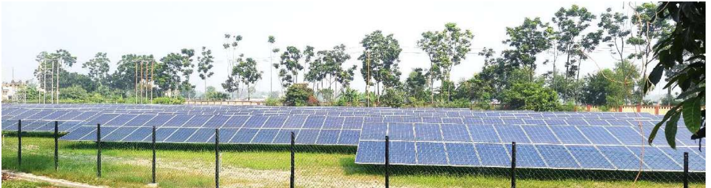
01 MWp Solar Power Plant at residential township
