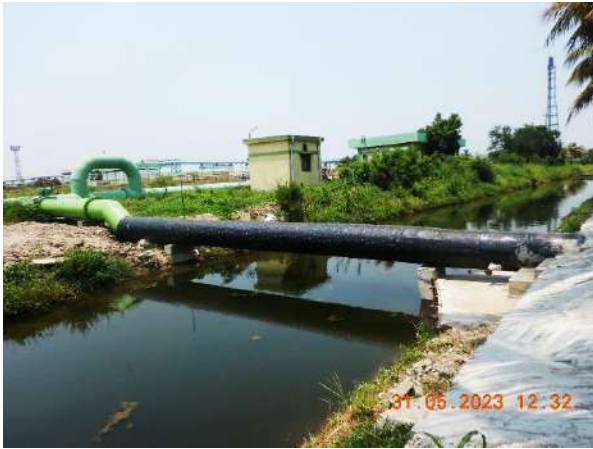
Discharge of treated effluent outside plant through pipeline without mixing into storm water
