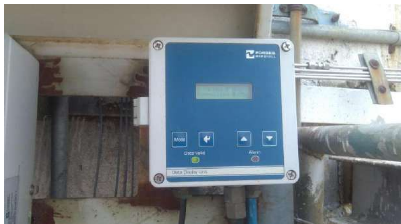
Online Flue Gas Monitoring System at CFB Stack
